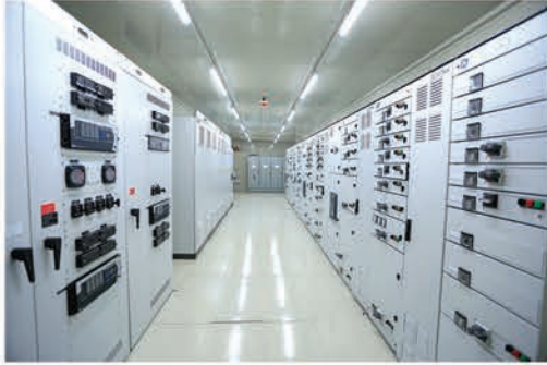
E-House Inside View
